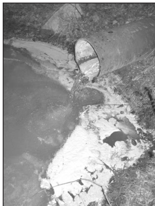
Sewage flows from an uncapped, abandoned City of Rome sewer line into Dozier Creek.
